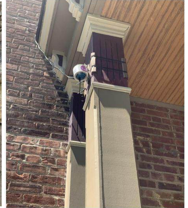
Kingston Public Library Purple Air Install
